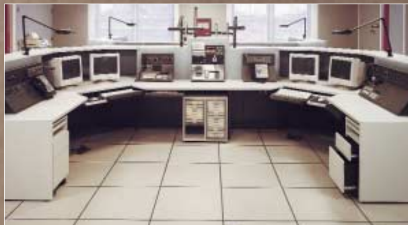
▼ The Geneva with adjustable twin vertical arm is installed in the command center.
